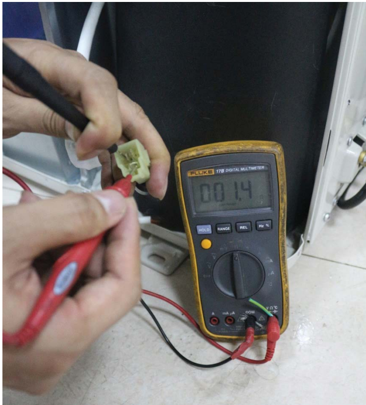
Fig. 55 – Test the voltage
