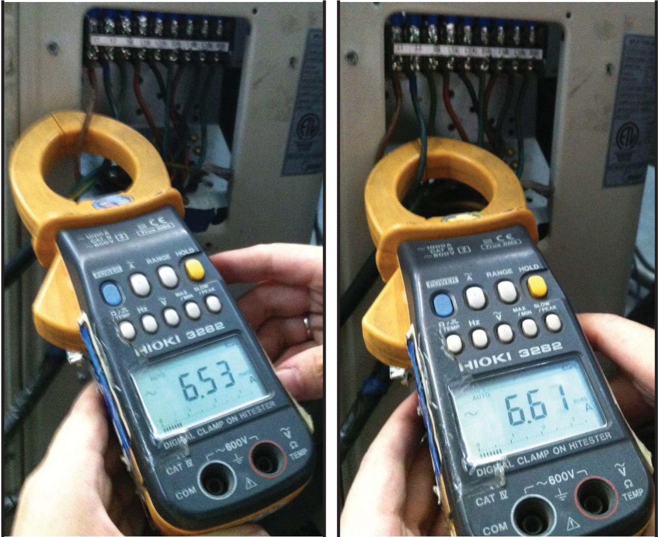
Fig. 53 – Test the voltage
