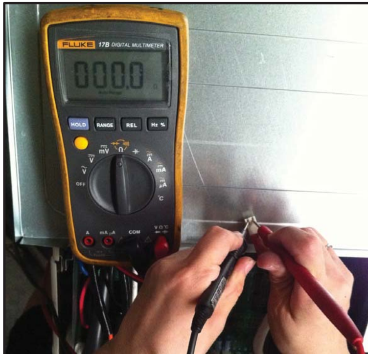
Fig. 50 – Test the voltage
